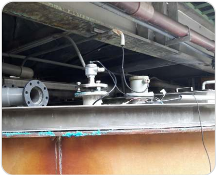
Copper sulfate storage tank
