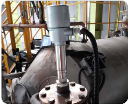
High temperature boiler
